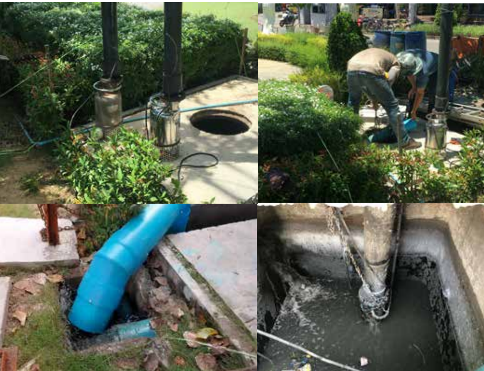
▲ Water Pump site: water drainage system for Suksan Village
